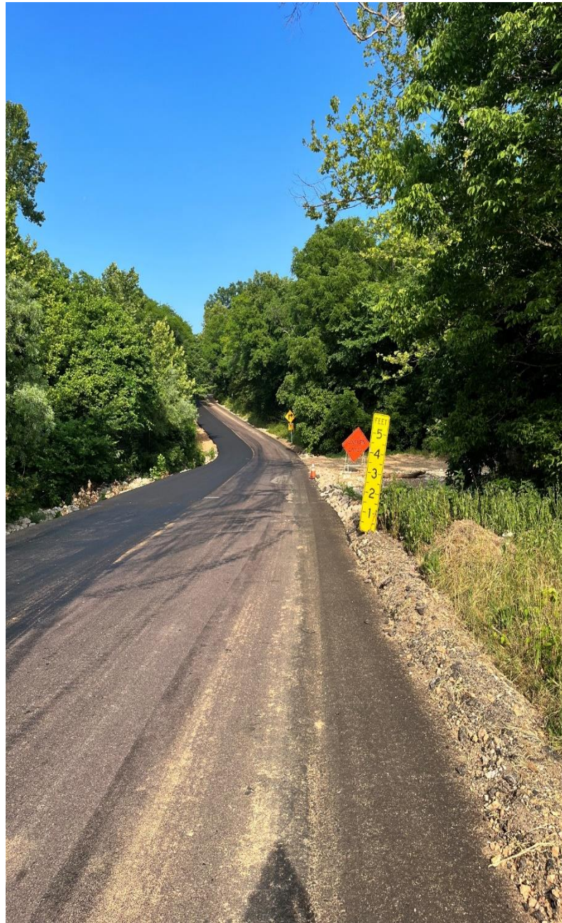
Figure 3.3 Area of Periodic Flooding
