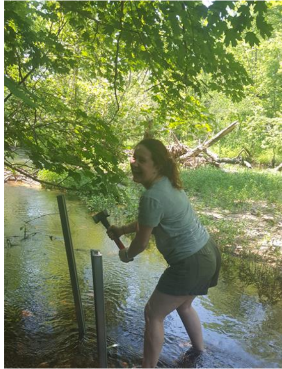
Figure A.42 Installation of SuperStruts Into a Streambed by the Author, T.N. Mortensen.
