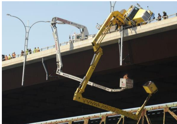
Figure 1.5. Snooper Truck Tipped Over onto Siderail [9]
