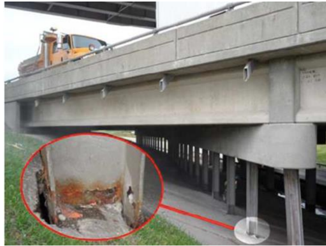
Figure 2.1: Corrosion of H-piles in I-70/I-270 interchange in St. Louis.
