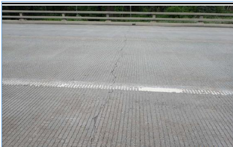
Figure 2.3 Cracks on silica fume deck at Troublesome Creek Bridge (Alaska DOT&PF Bridge Section, 2018)
