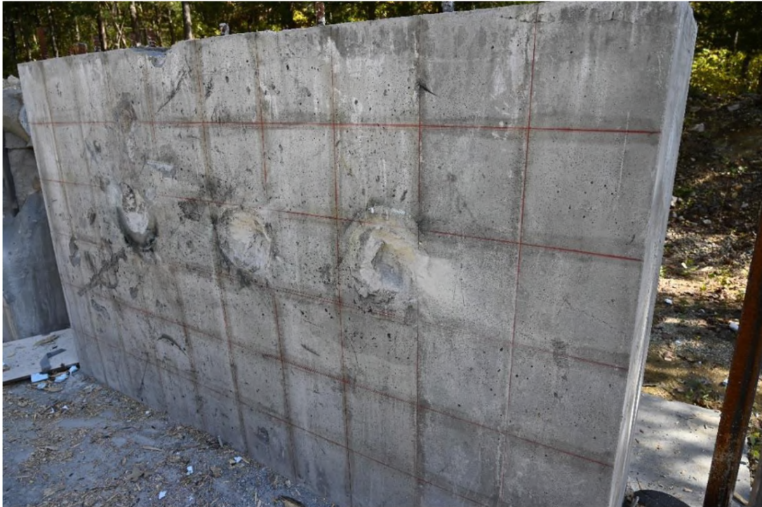
Figure 5.8 Reinforced 120 psi Seal Damage
