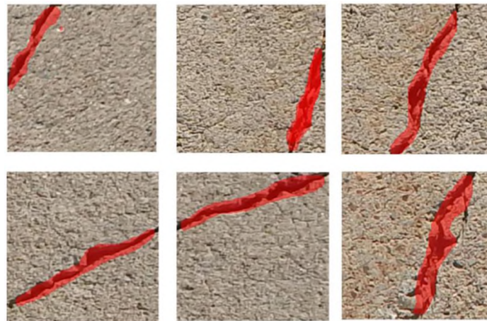
Figure 4. Examples of detected cracks with the deep learning algorithm
