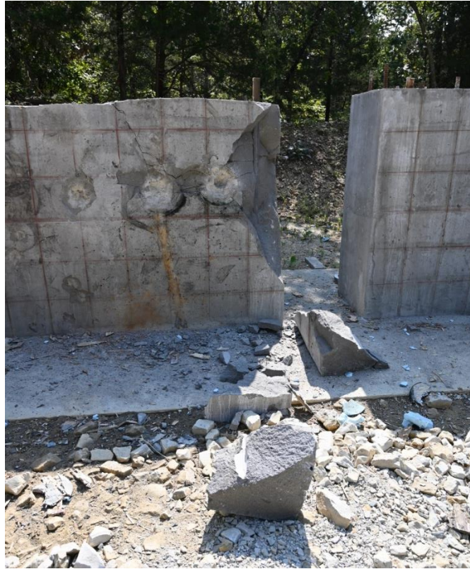
Figure 3.6. 50 psi seal catastrophic failure
