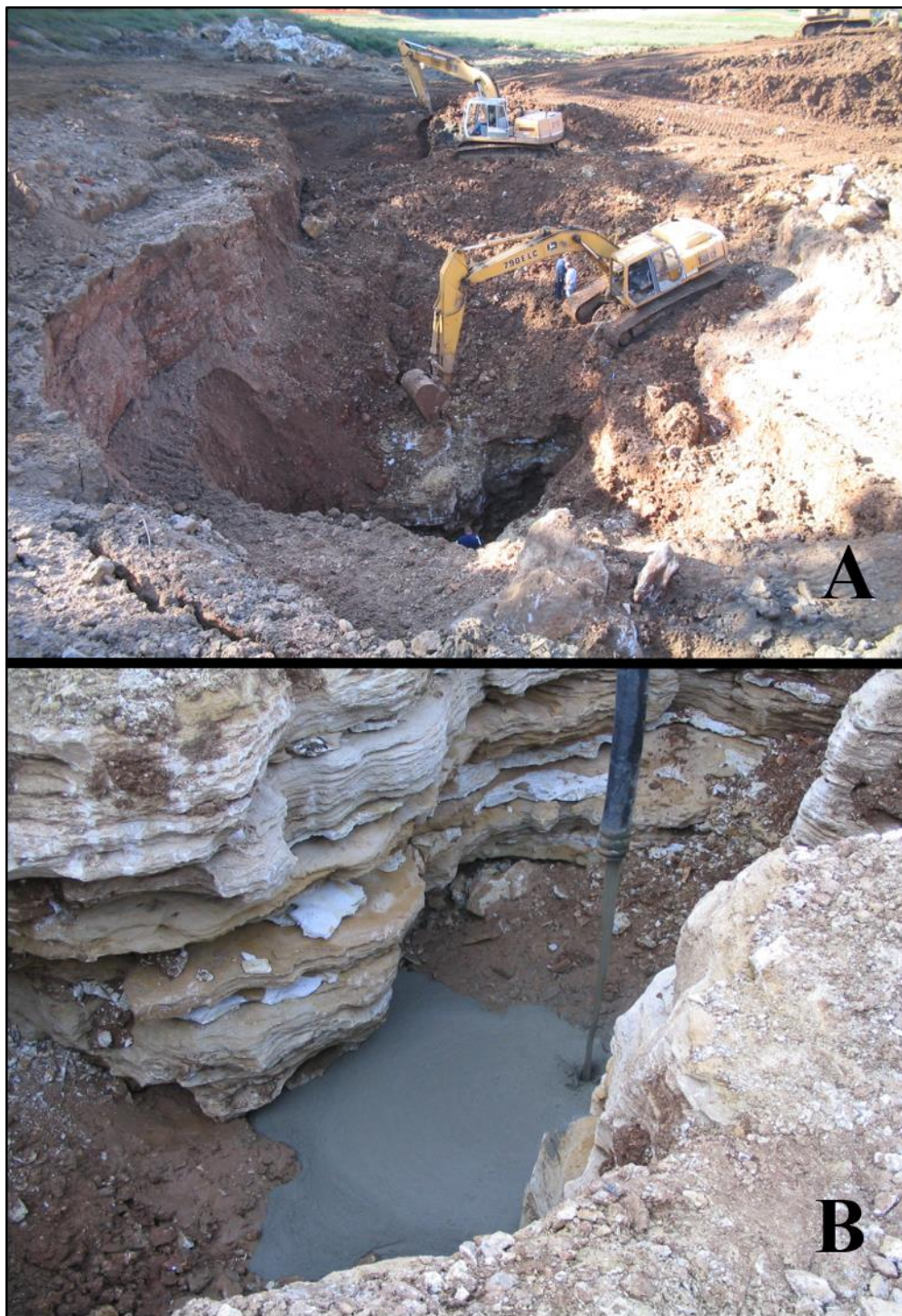
Figure 1.4. Photo A and B of 2004 sinkhole and remediation. A: Looking south along Lake Chesterfield, showing scale of the sinkhole and remediation. B: Sinkhole being filled with grout, in this photo you can clearly see the highly weathered limestone (Wieners, 2005).
