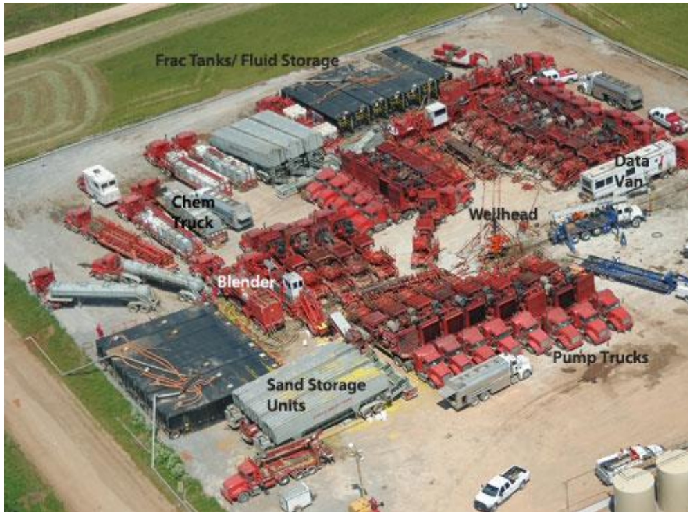
Figure 2.1. Surface facilities of hydraulic fracturing operation
