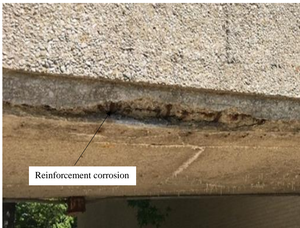
Figure 1.3. Bridge deck deterioration shows reinforcement corrosion.
