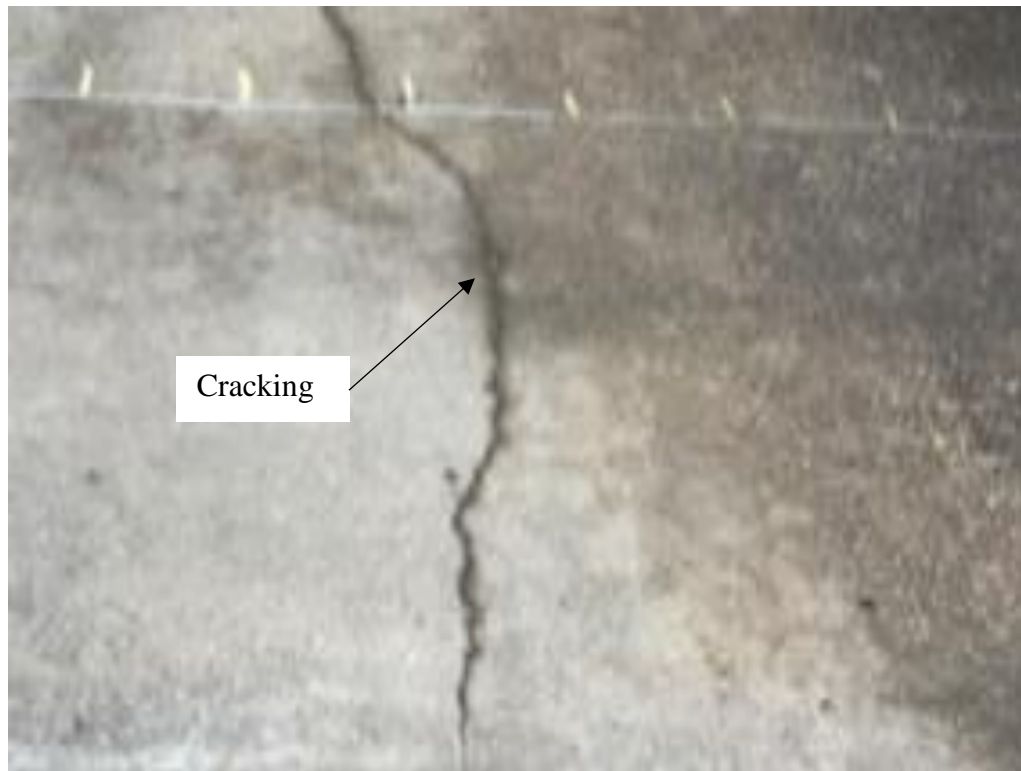
Figure 1.6. Bridge deck deterioration shows cracking.
