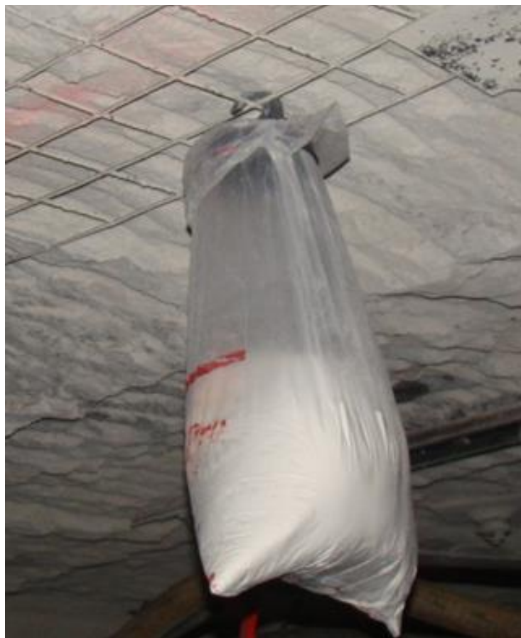
Figure 4.9: Barrier Bag Hung from Roof Mesh
