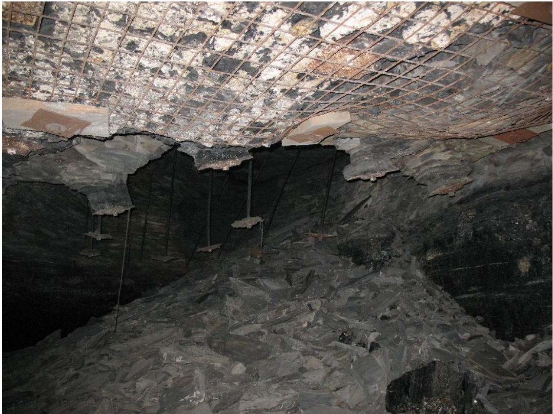
Figure 1.2: Large rock layer that has fallen inside a mine (Molinda and Mark 2010).
