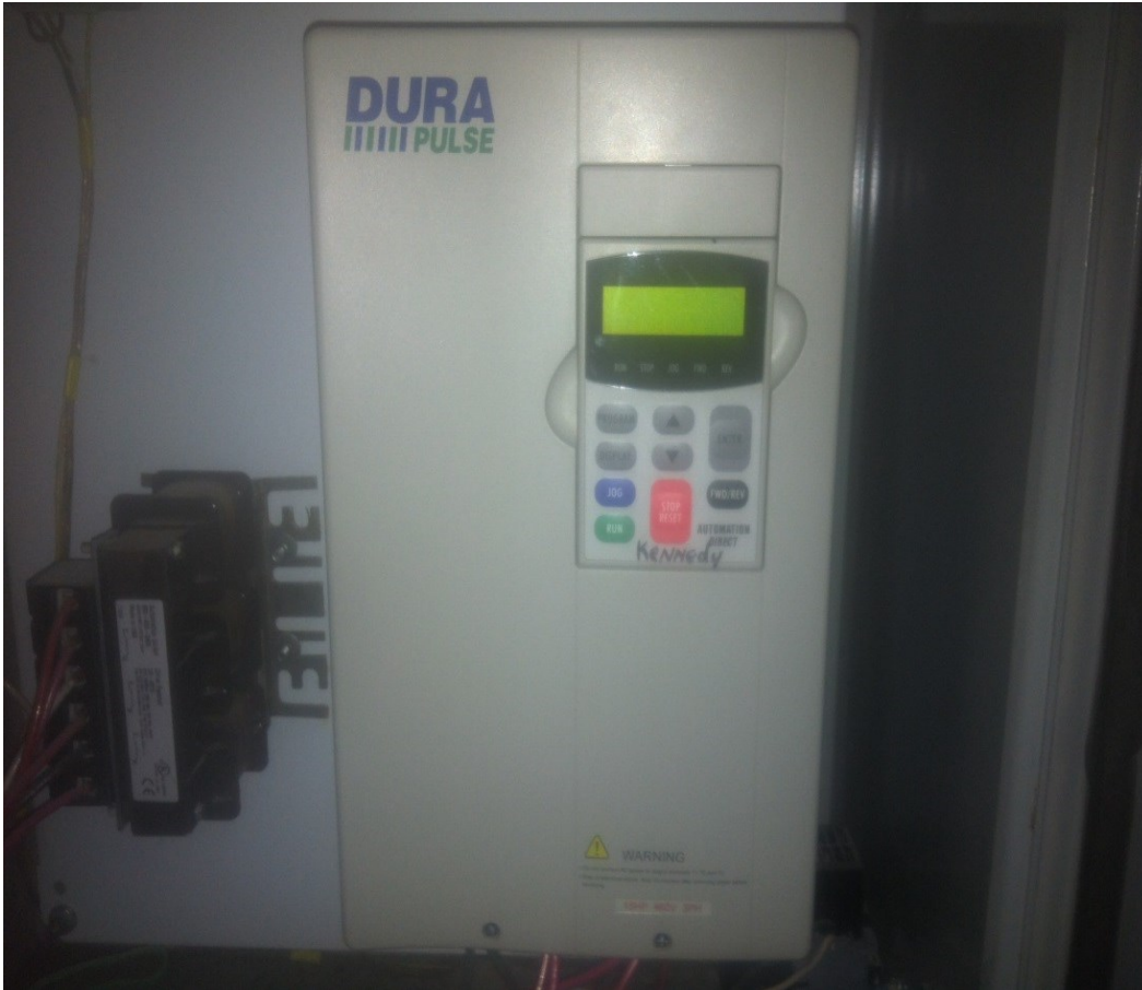
Figure 3.12 Variable frequency drive
