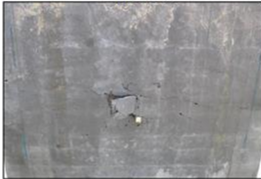
Panel 3 rear surface after explosion - Very slight scabbing at the surface of the panel. - Minor cracks through the panel. - Structurally undamaged.
