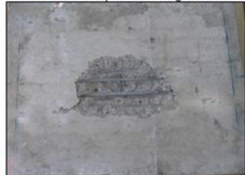
Panel 4 rear surface after explosion - Heavy scabbing, reinforcing bars exposed. - Cavity approximately 480 mm x 300 mm, with a maximum depth of 50 mm (1/2 section depth).
