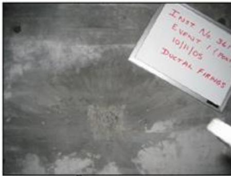
Panel 3 (Ductal ® ) front surface after explosion No cracks
