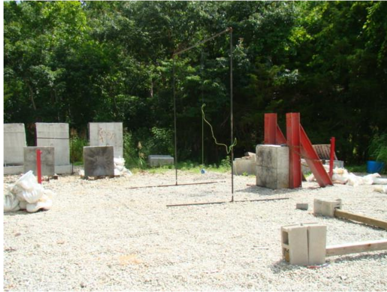
Figure 6.1 Barrier chained to supporting I-beams
