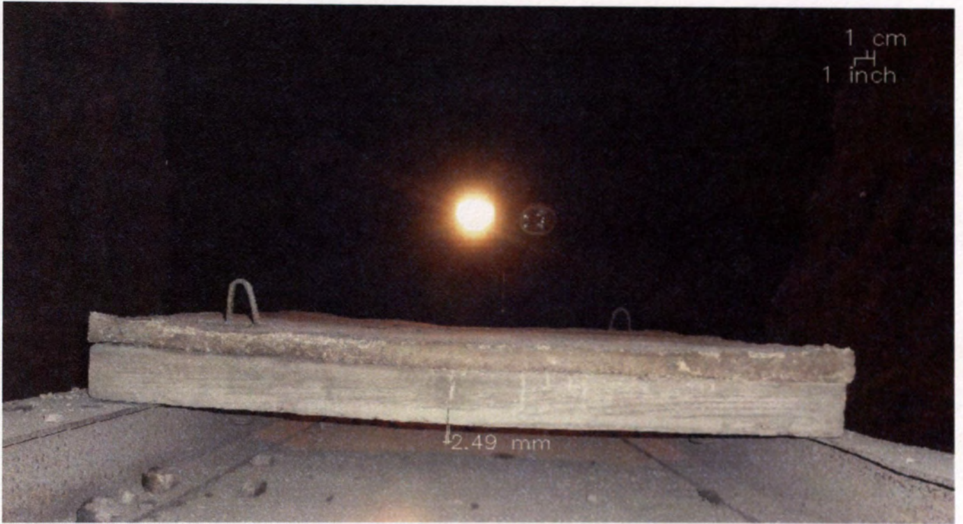
Figure E.8 – Flexural Cracks in the Back Face of 2-H, 1 st Event
