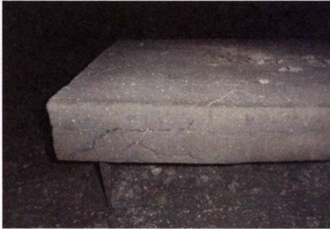
(c) Shear Cracking Front Face
