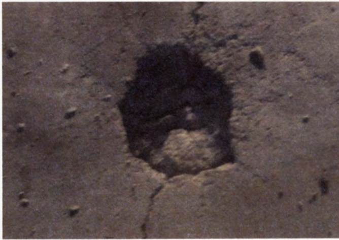
(c) Punching Failure
