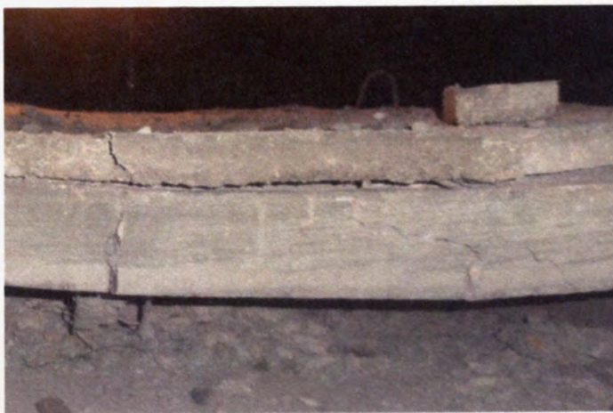
(e) Flexural Cracks in the Back Face
