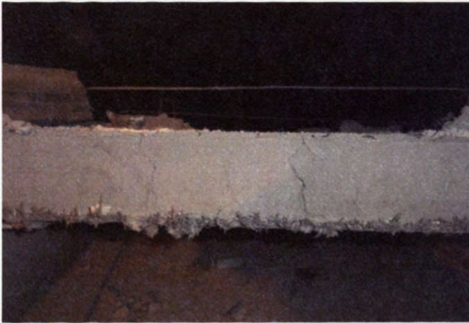
(c) Flexural Cracks Front Face
