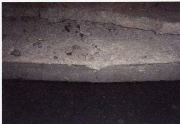
(e) Large Crack Back Face of Panel
