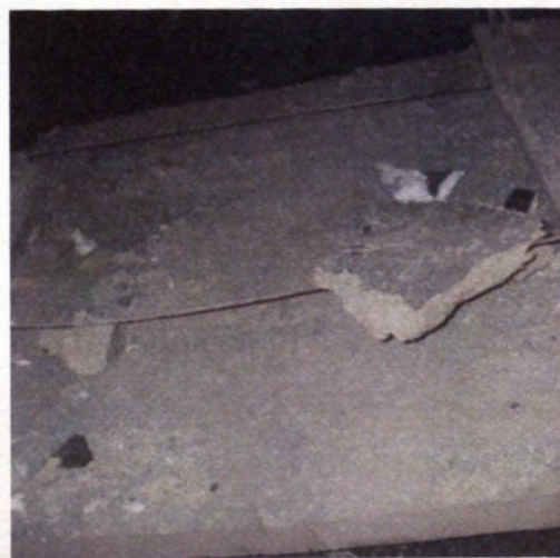
(e) Compression Face After FA-WF Pieces were Cleared Off
