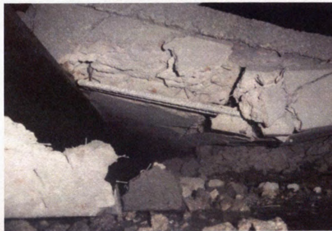
(e) Crack and Debris From Front
