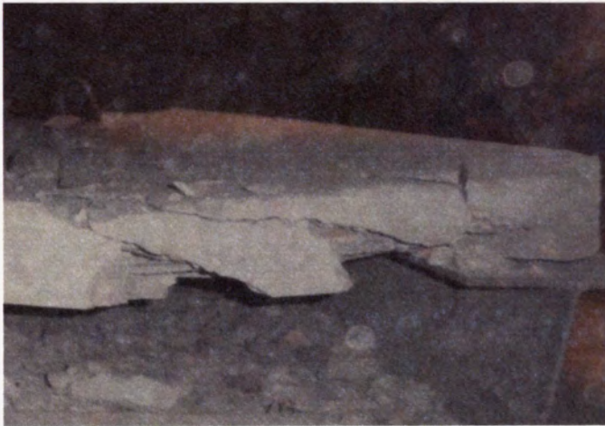
(c) Shear Crack in the Front Face
