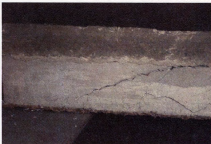
(c) Shear Crack in the Front Face
