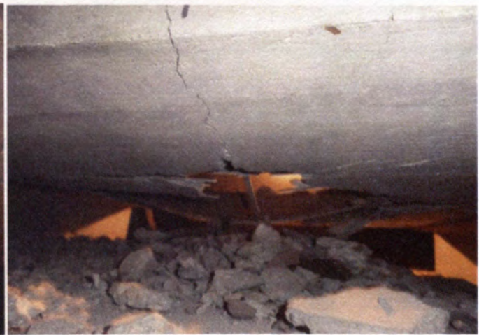
(f) Debris and Tension Face
