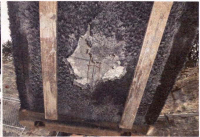
(f) Exposed Rebar and Chair Tension Face
