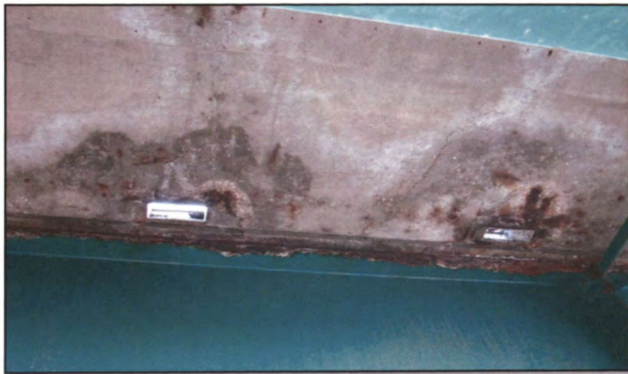
(b) Deterioration due to unguttered water drainage.
