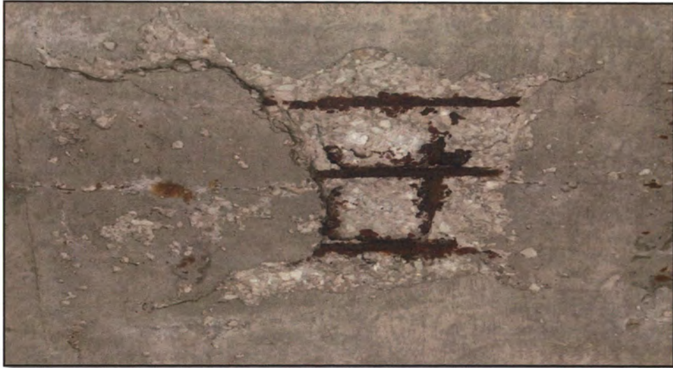
(a) Example of severely deteriorated bridge slab.
