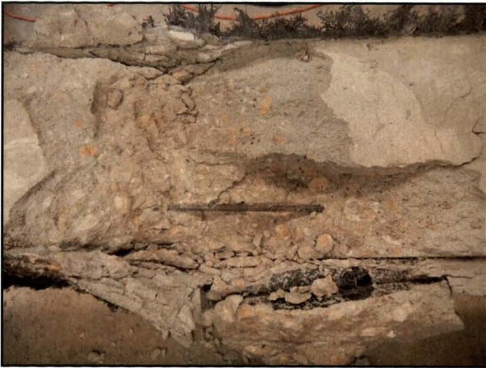
Figure 4.9. Top View of Failed Test Beam F-P-A-L
