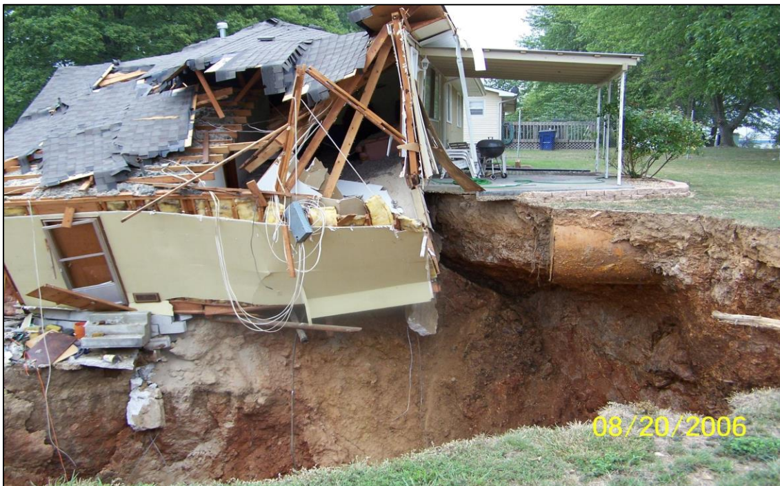
Figure 1.1. 2006 Photograph of a collapsed sinkhole with a damaged house in Nixa Missouri (Anderson, 2006).
