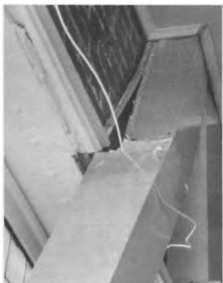
Fig. 16 Buckled Brace in URM Building
