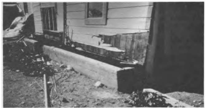
Fig. 2 Damage to House Not Bolted to Foundation
