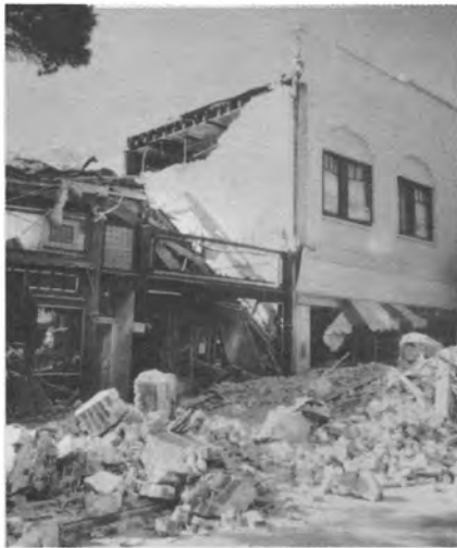
Fig. 8 Masonry Wall Fell on to Adjacent Roof
