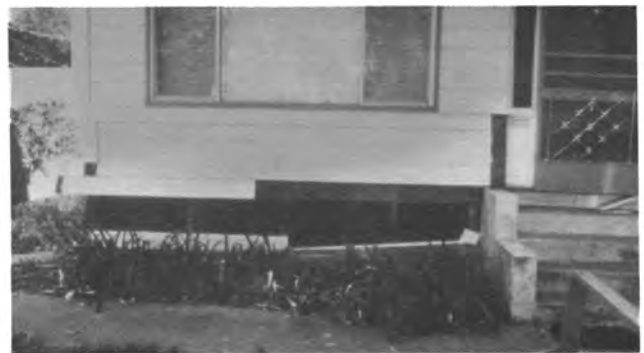
Fig. 3 Damage to "Pony" Wall
