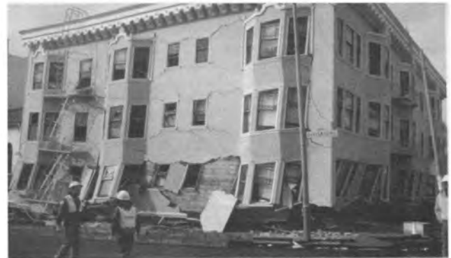
Fig. 5 Collapse of Apartment in Marina District
