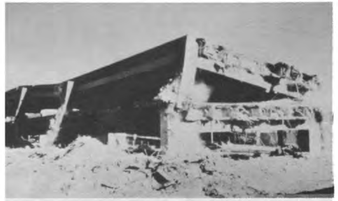
Fig. 23 Failure Mode Observed during Demolition
