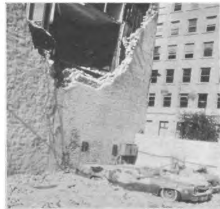
Fig. 7 Out-of-Plane Failure of Masonry Wall
