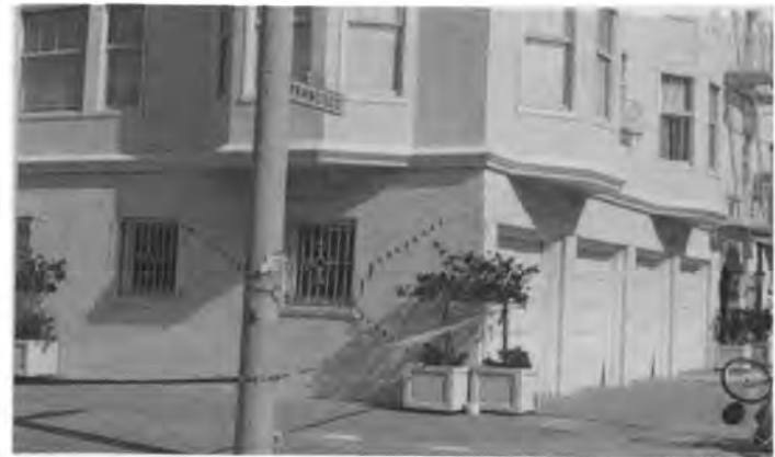
Figure 16. Marina district, San Francisco, October 24, 1989. View north east from junction of Divisadero and Francisco, showing damage due to shaking along Divisadero.
