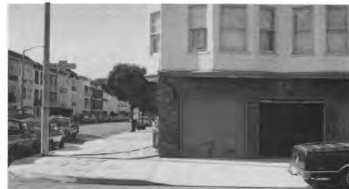
Figure 17. Marina district, San Francisco, October 24, 1989. View north from junction of Broderick and Bay, showing damage due to shaking along Broderick.
