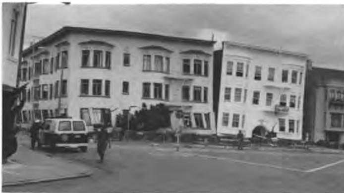
Figure 14. Marina district, San Francisco, October 24, 1989. View north east from junction of Prado and Cervantes showing damage due to shaking along Cervantes.
