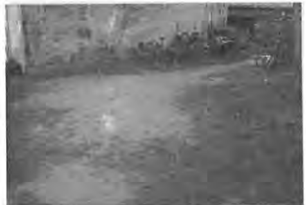
FIG. 4 Sand Boil, Bihar P.W.D. Rest House, Darbhanga.
