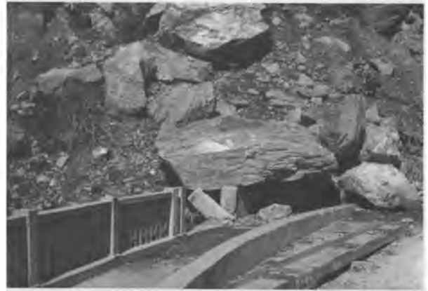
FIG. 12 The Damaged Railings of the Legship Bazar Bridge.
