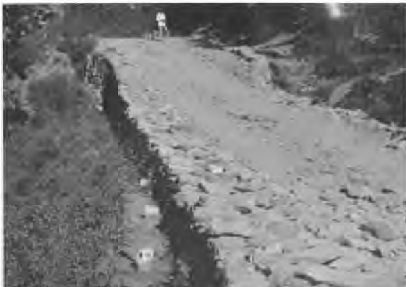
FIG. 15 Subsided Stretch of Gangtok-Legship State Highway (partly repaired).
