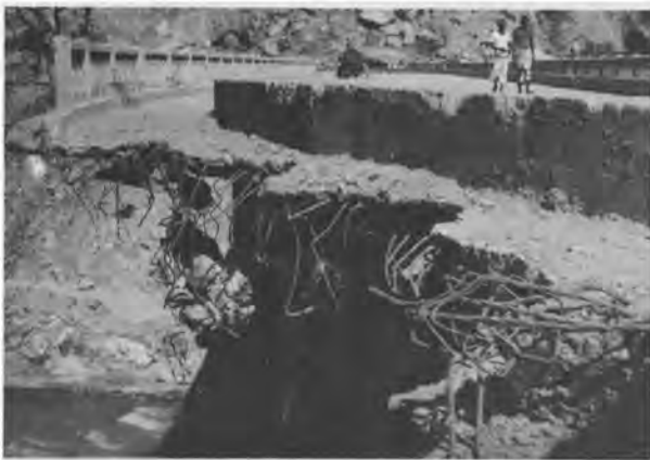
FIG. 11 The Damaged Deck of the Legship Bazar Bridge.
