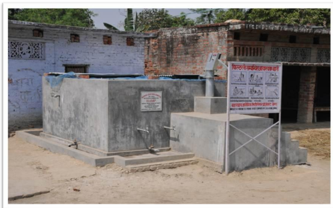
Fig. 15. Photo of Gravel Sand Filter (GSF) in the village
