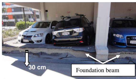
Fig. 13 Building on pile foundations in area of severe liquefaction showing large settlement of the surrounding soils relative to the foundation beams
