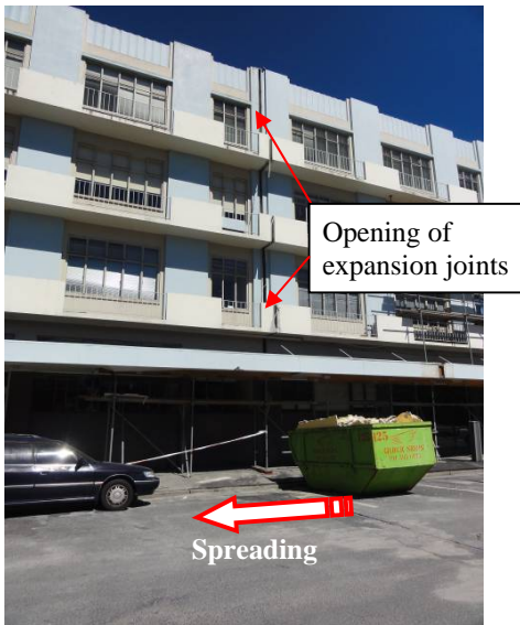
Fig. 14 Stretching of foundations due to lateral spreading resulting in opening of the expansion joints of a CBD building
