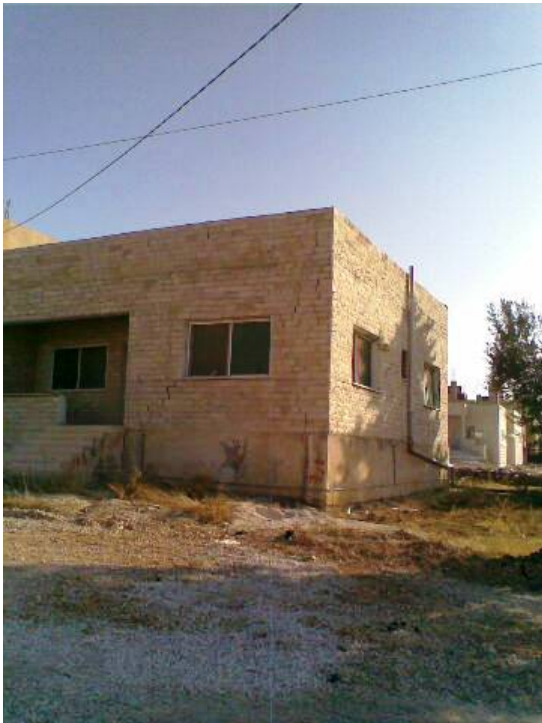
Fig: 3 Damaged Building: evacuated damaged portion
