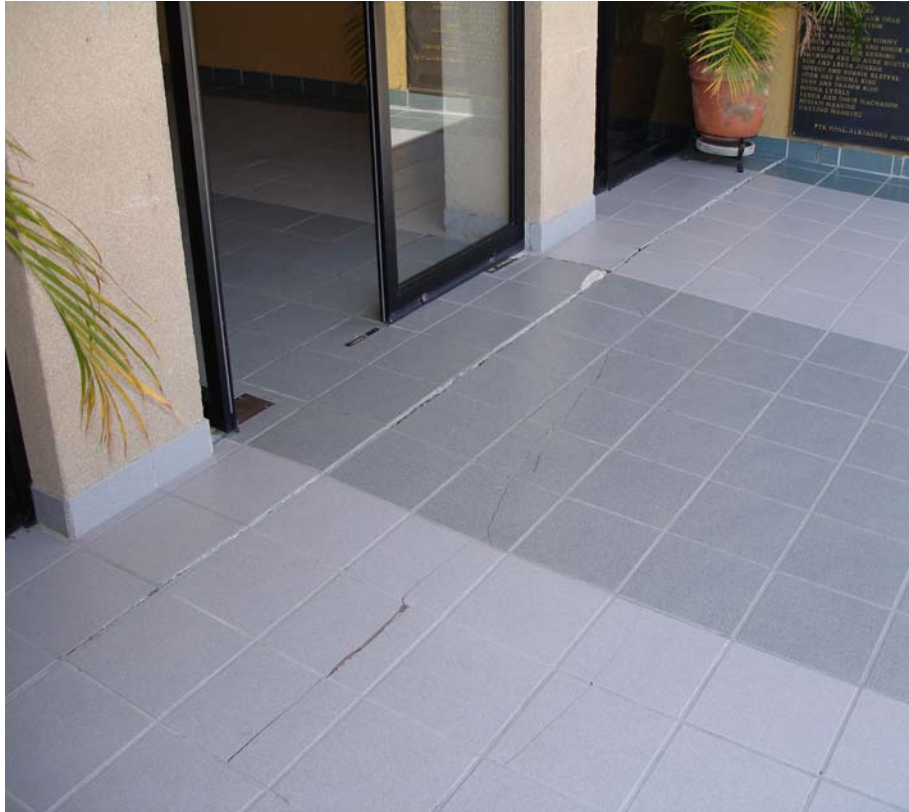
Fig.3 Cracking and deformation on the floor.
