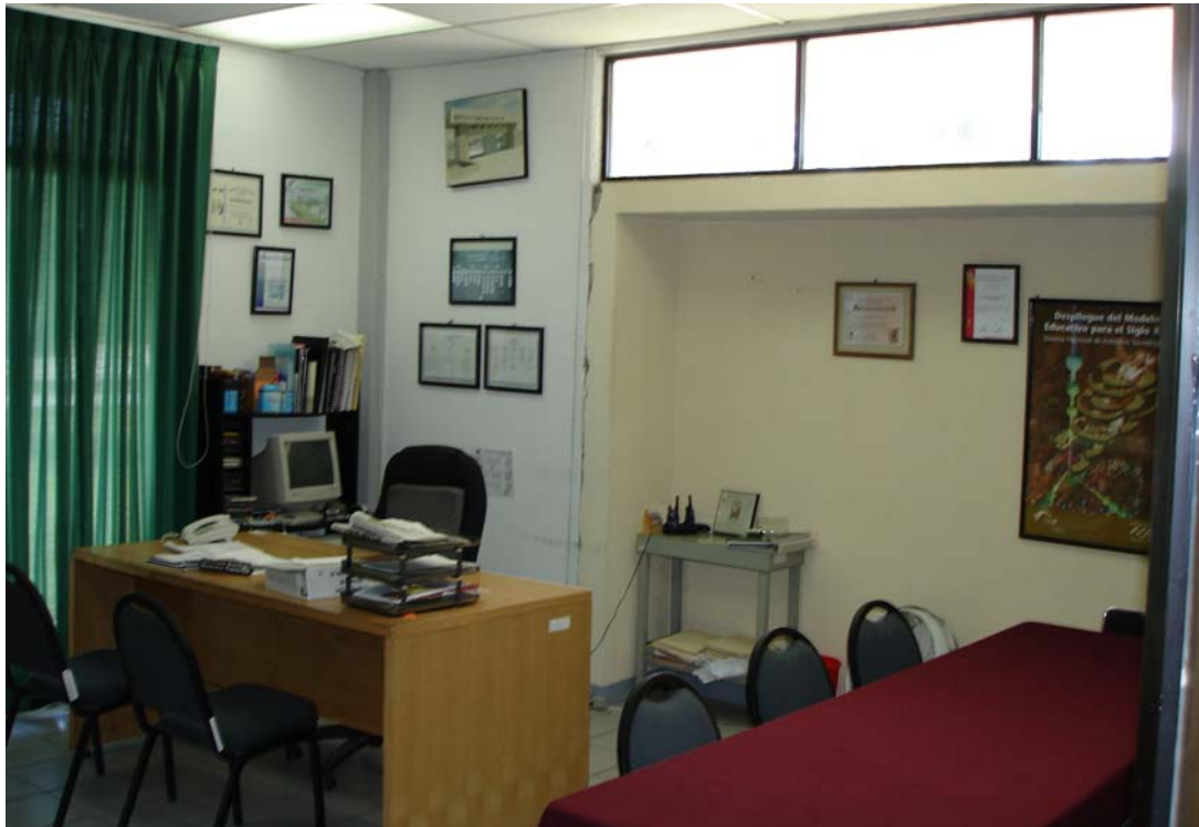
Fig.4 Vertical cracking joint between the wall and the column in the library cubicle.
