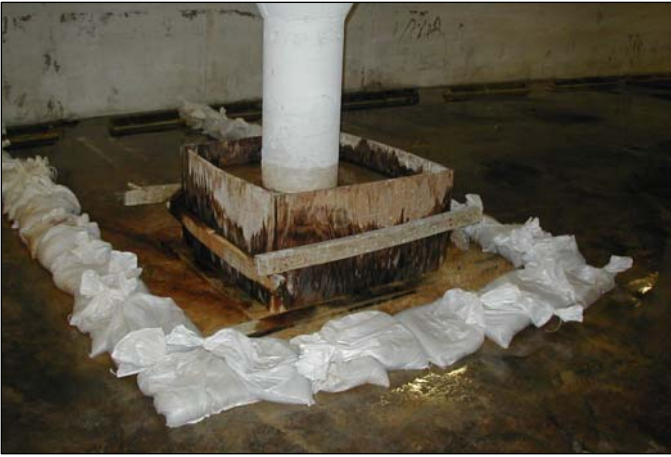
Photograph D – Observed seepage within subterranean level
