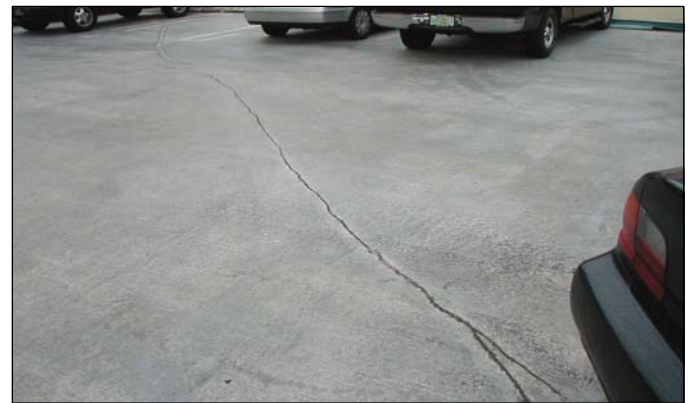
Photograph B – Observed cracks on elevated deck
