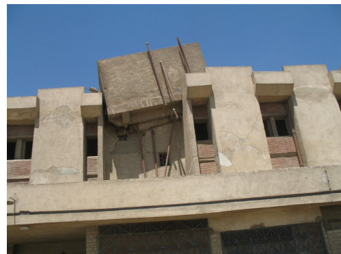
Photo 3 Failure of tank at the roof
