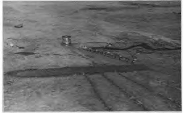
Fig. 11 - Test Setup of Passive Isolation by a Soil-Bentonite Trench (Site 4 with barrier)
