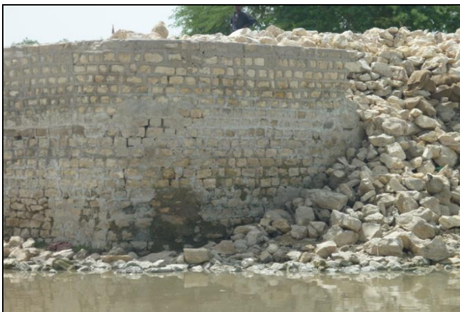
Fig.20 Stone masonry flood protection embankment at a critical location showing poor construction quality (Amir, 2010)
