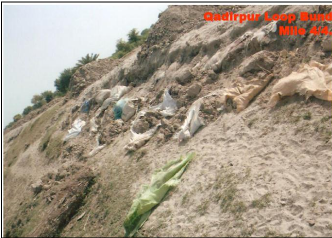
Fig.19. A rehabilitated flood protection embankment showing fate of construction material and quality of embankment to face future floods (Amir, 2010)
