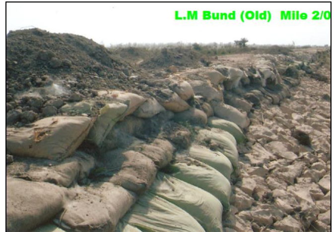
Fig.17 Flood protection embankment; an evidence of inadequate construction material and poor finished quality (Amir, 2010)
