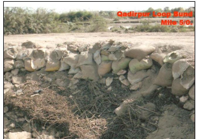
Fig. 18 Flood protection embankments with inadequate construction material and poor finished quality (Amir, 2010)
