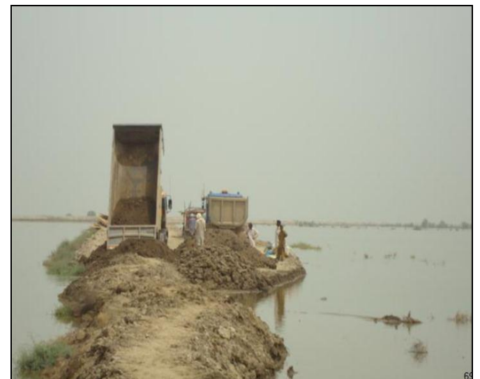
Fig.23 Rehabilitation of embankment of RBOD for future floods, the material and method adopted makes its efficacy doubtful (Amir, 2010)
