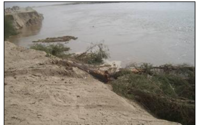
Fig.22 Fate of earthen embankment of RBOD during 2010 floods (Amir, 2010)
