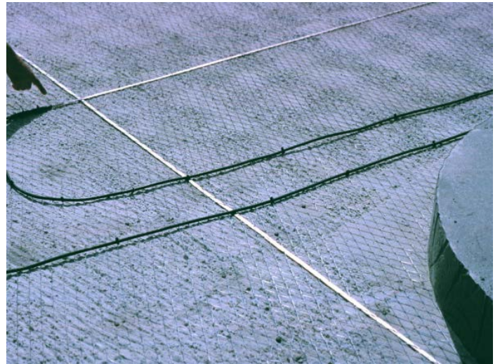
Fig. 8: Cathodic Protection System
