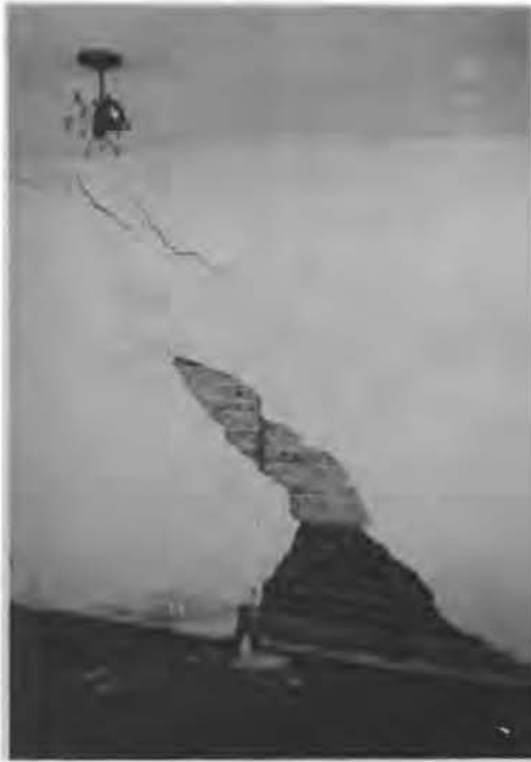
Fig. 2 Typical Cracking Due to Settlement
