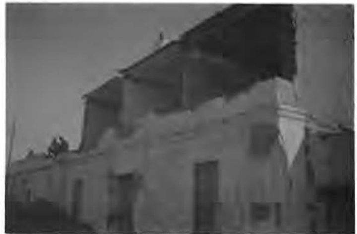
Fig 7 Collapse of Outer Walls of a Two Story Adobe Building
