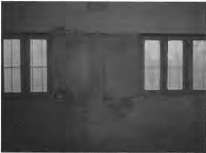
Fig 5 Shear Failure of a Short Column Arising due to the Existence of Large Windows.
