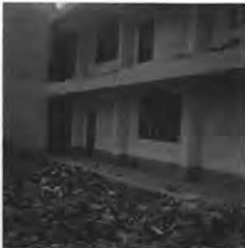
Fig 6 Failure of Parapets due to the Absence of Lateral Support
