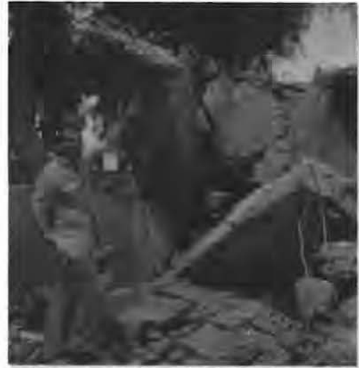
Fig 3 Widely Spaced Stirrups and Smooth Cold Joints
