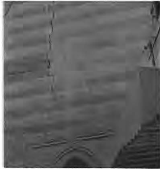
Fig 9 Wall Cracks of El-Sultan El-Ghoury Mosque
