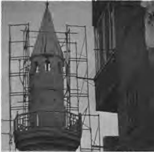
Fig 8 Damage of the Minaret of El-Hady El-Yousefy Mosque
