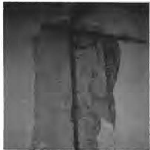
Fig 4 Separation of Buildings and Column Damage Due to Pounding
