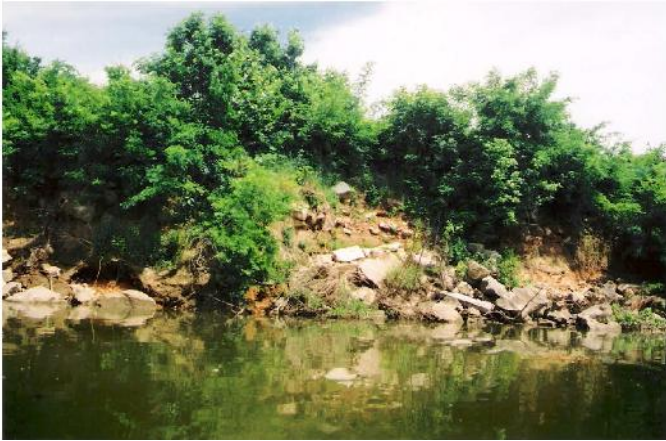
Fig. 6. Failed slope in east bank of river 210 ft south of intake pipeline
