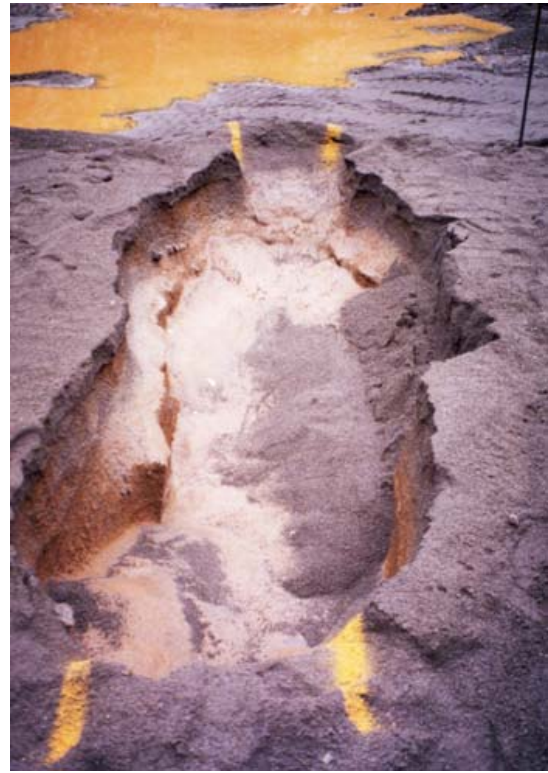
Fig. 7. Trench wall collapse in filter embankment after flooding
