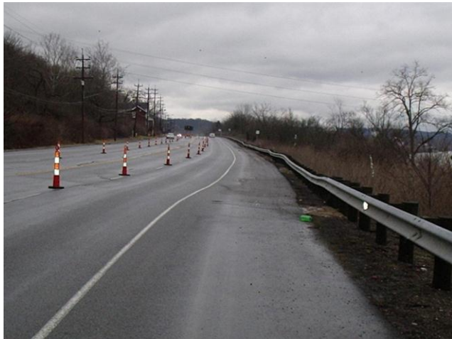
Fig. 16: Road damage in 2005 (pre-repair).
