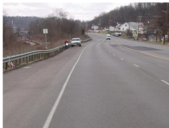
Fig. 1: Pre-repair road distress (2005).
