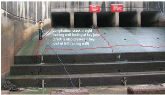
Figure 28 – Addicks Dam Parabolic Chute Slab with Existing Longitudinal and Transverse Cracks
