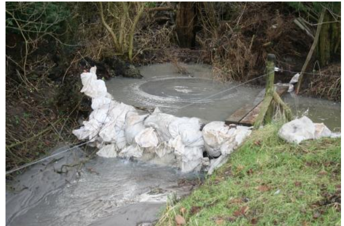
Figure 5: Sand boil surround by sand bags (Picture by Laurens Pompe, Waterschap Rivierenland)
