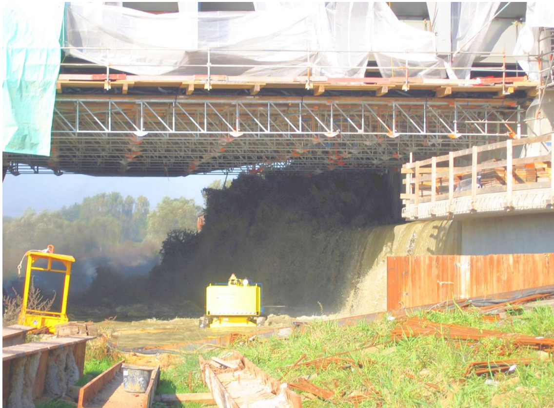
Fig. 6: Violent water flow through the two abutments into the Lippe River
