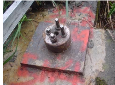
Fig. 10 (b) Tendons uneven shrink caused by angular bending
