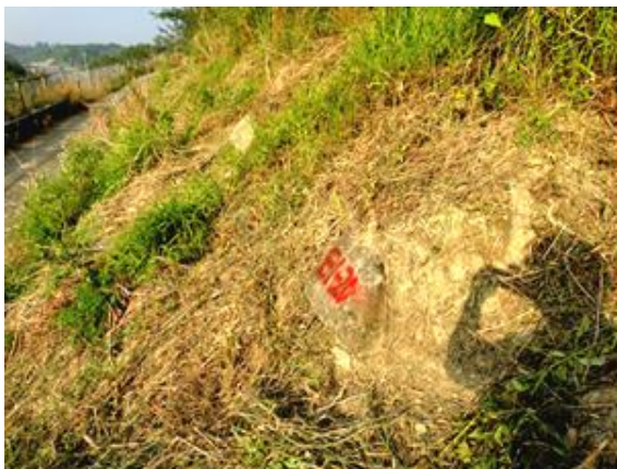
Fig. 12 (a) Anchor head sink in creep soil
