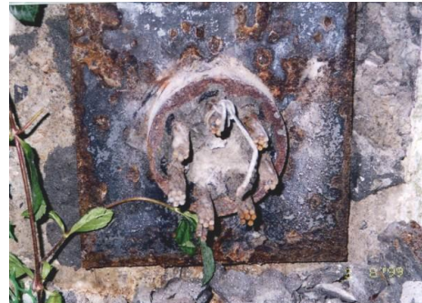
Fig. 11 (a) Anchor head corrosion
