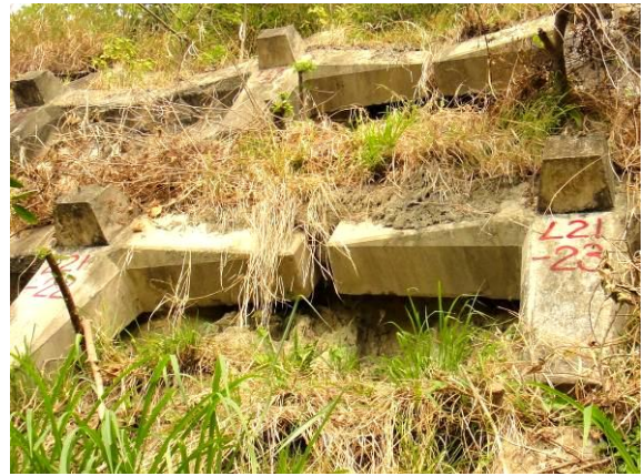
Fig. 12 (b) Topsoil hollowed Fig. 12 Prestressing lose conditions
