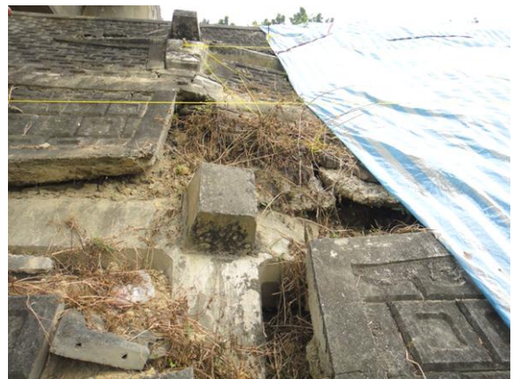
Fig. 13 (a) Prestressing load increase because of slope sliding
