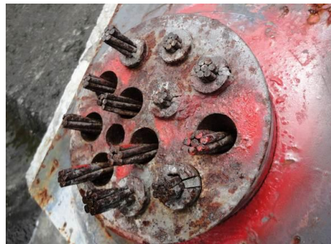
Fig. 11 (b) Tendons shrink ; Corrosion of anchor head and the wedges slip
