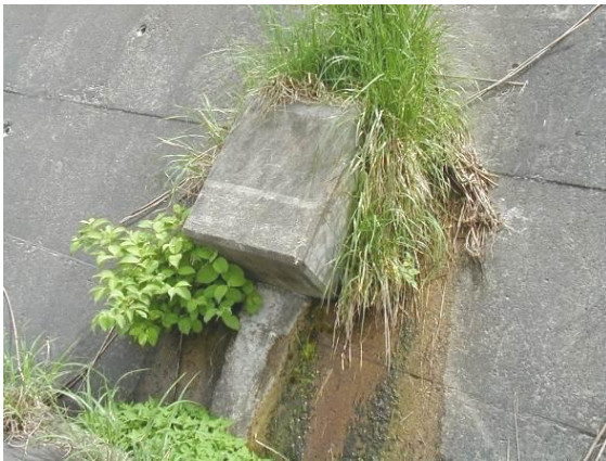
Fig. 11 (d) Efflorescence or groundwater seeping out Fig. 11 Anchor head corrosion and wedges slip and breaking of tendons
