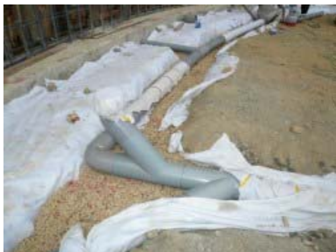
Fig. 4. Drainage System Photo - Hsinchu
