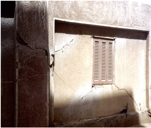
Photo 2. Cracks observed at light structures
