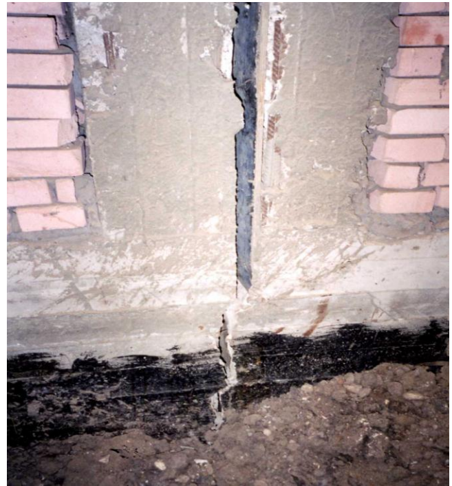
Photo 1: Cracks observed at foundation elements.
