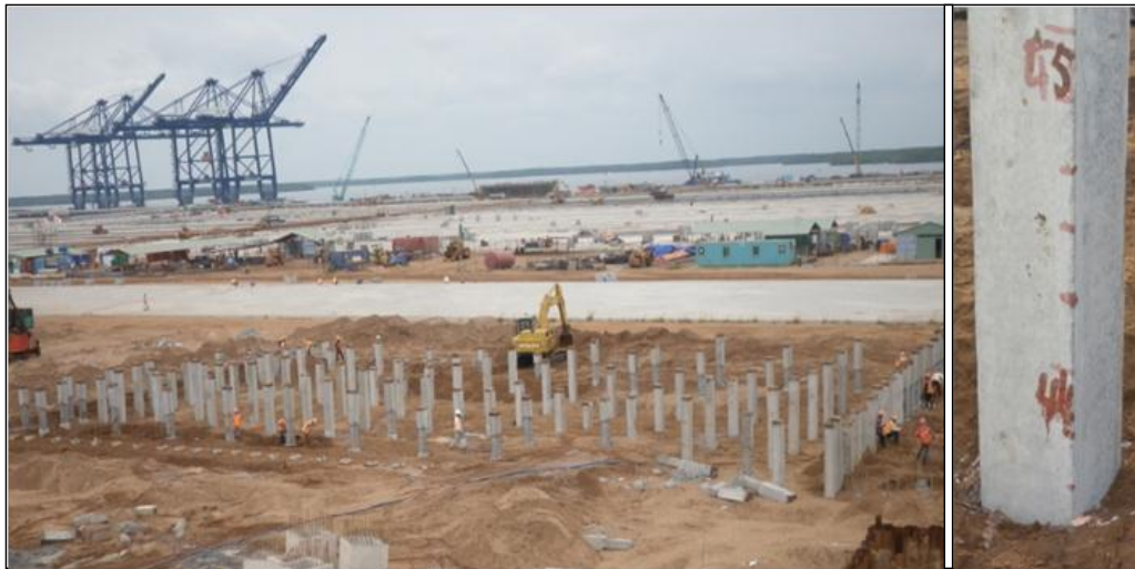
Fig. 10. View on Feb. 10, 2012, of the Maintenance Shop area with about half the piles lengthened (Authors' photo)
