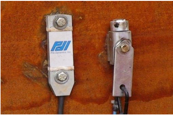
Fig 3. Installed Strain Gauges (left) and accelerometer (courtesy of CPR Asociados)
