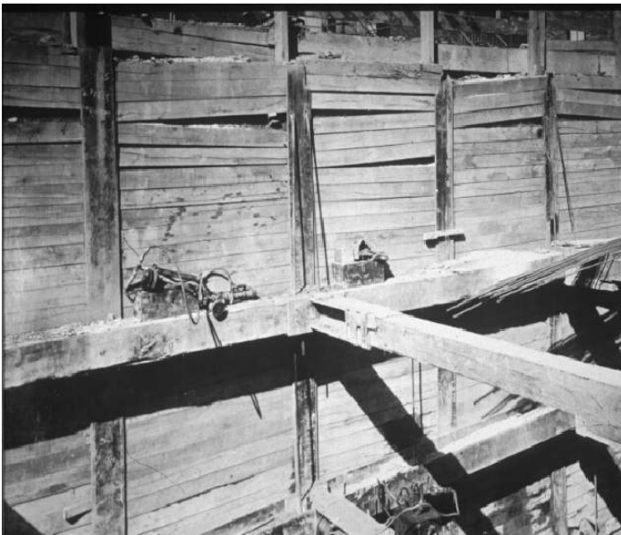
Fig. 3. Close up view of steel H-piles, timber struts, steel walers and timber lagging used to support an open cut of the Chicago Subway, as seen in 1940. Karl Terzaghi wanted Peck to measure strut loads to see if clays adhered to the wedge theory of lateral soil pressure for sands he had proposed after studying the Berlin Subway collapse in 1936.
