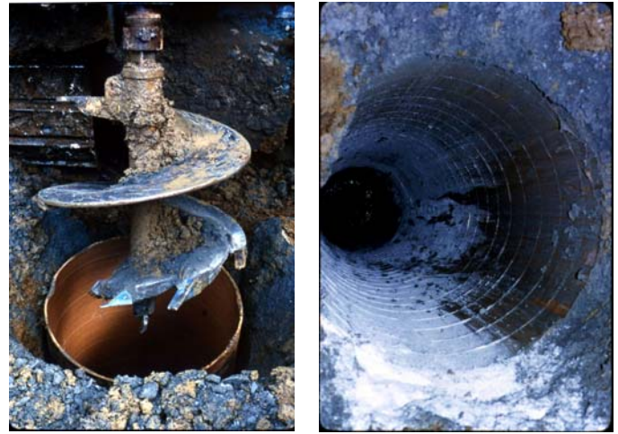
Fig. 13. Photos of 24-inch diameter augered caissons being excavated at the course project site along The Embarcadero in San Francisco, in September 1977. The contractor chose to employ Sonotube forms as temporary casing, using lime to improve working conditions on the excavated pad, which extended into soft estuarine clays.
