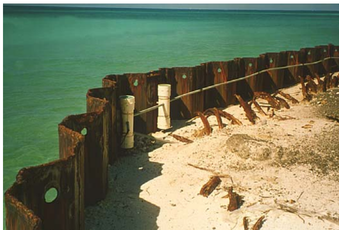
Fig. 15. Cathodic protection applied to steel sheetpile bulkhead wall on Sand Island Inner Harbor, Midway Atoll. Remnants of previous bulkhead wall can be seen behind the replacement structure.
