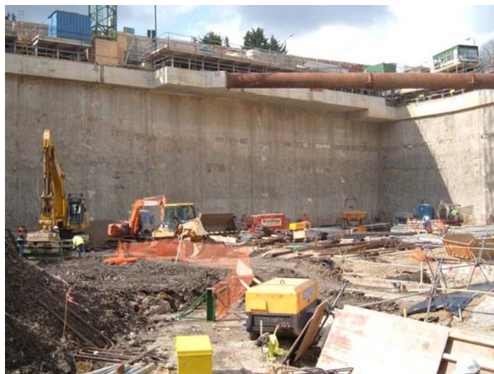
Fig. 11. Excavation of the basement for Kings Place Development (courtesy of Sir Robert McAlpine)
