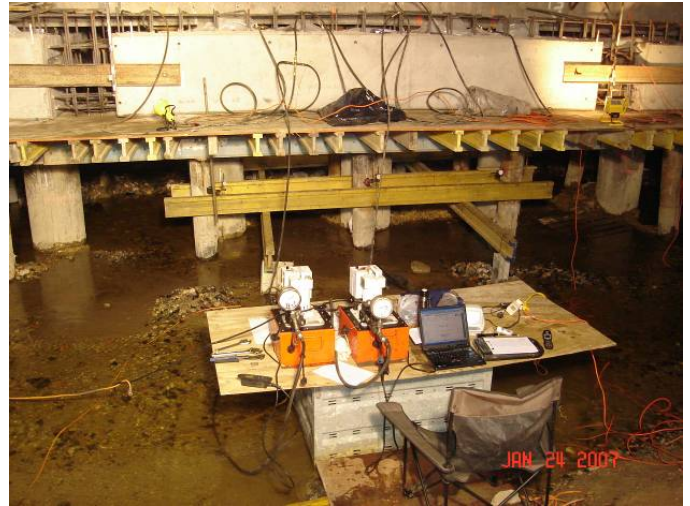
Fig. 10. Typical proof load test set up performed to a group of six micropiles.
