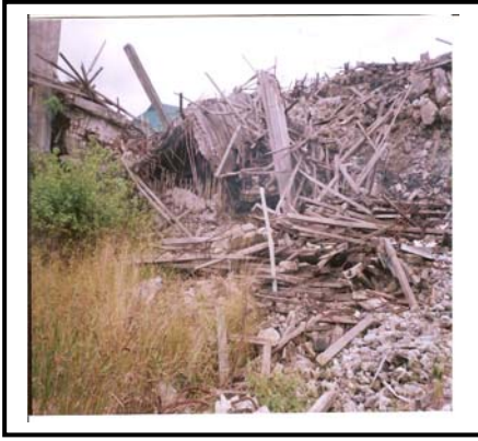
Fig. 6e: Remains of the collapsed building along the New Tombia Extension Road GRA III, Port Harcourt..
