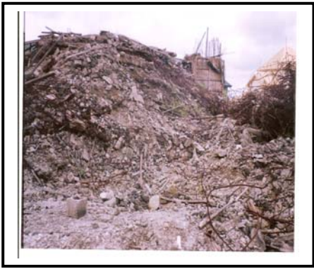
Fig. 6a: The collapsed building along the New Tombia Extension Road GRA III, Port Harcourt.
