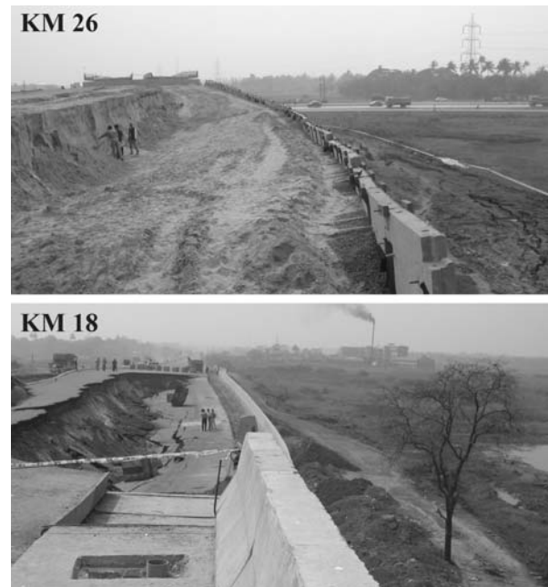
Fig.1. Failures at KM 26 and KM 18site.
