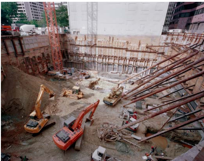
Figure 13: Site Excavation Completed Looking West at Supported Wall (copyright Dan Cunningham Photography)
